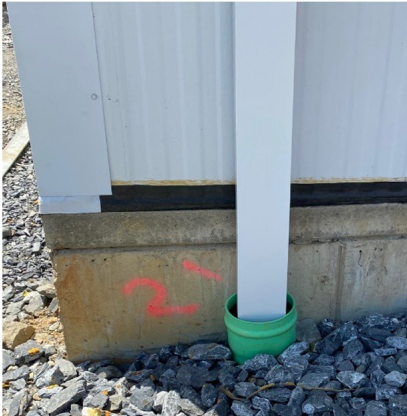
Rooftop gutters feed water to reservoir
